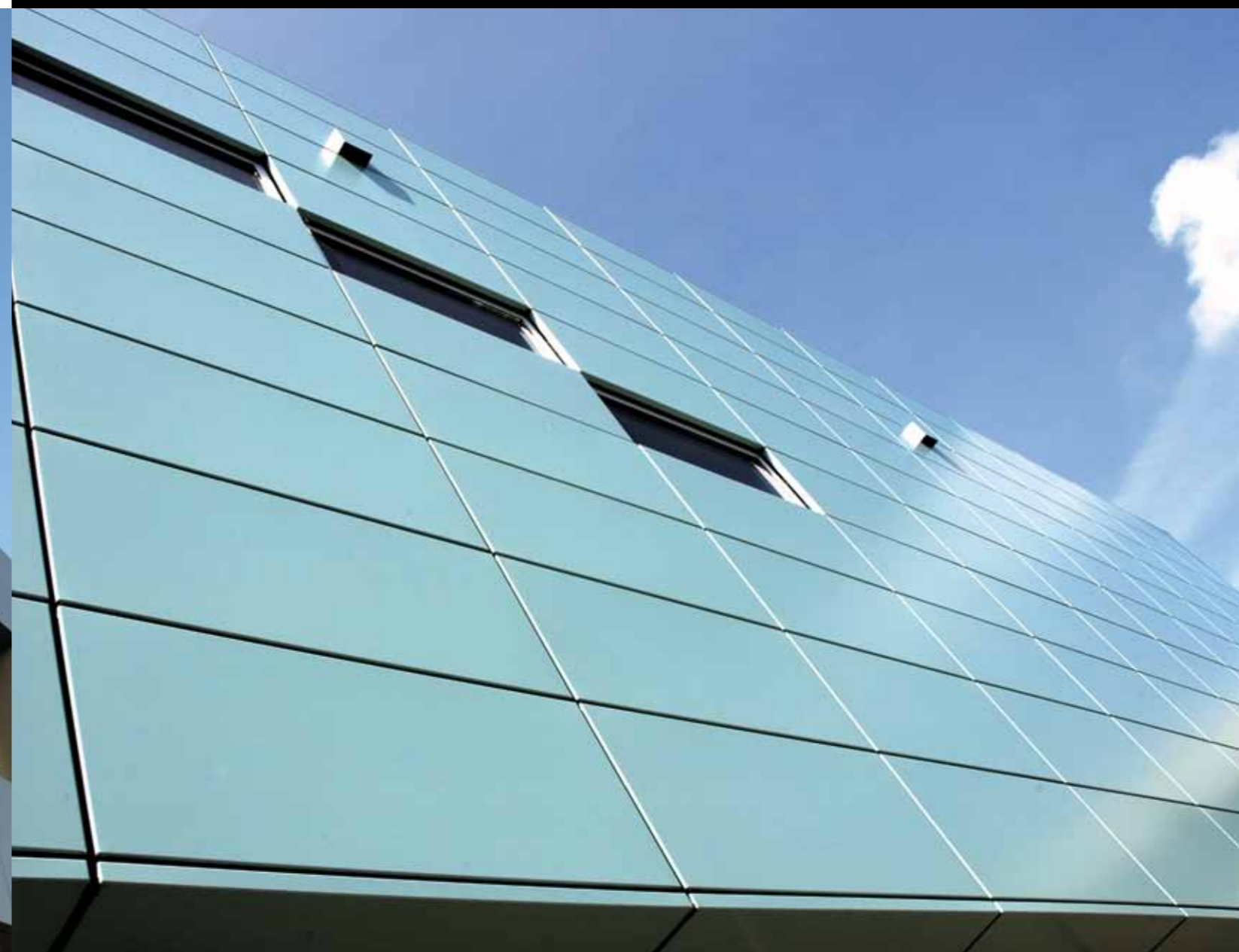
NKI-AVL Auditorium, Amsterdam (NL) | Architect: De Jong-Gortemaker-Algra, Rotterdam (NL) | Limeparts: aluminium powder coated
